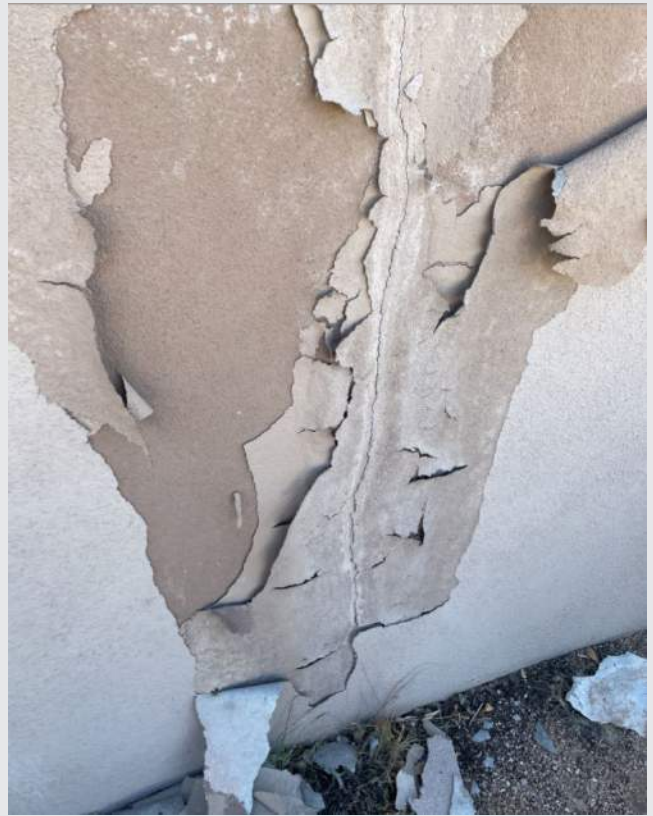
Layers of stucco repair and paint without underlayment
