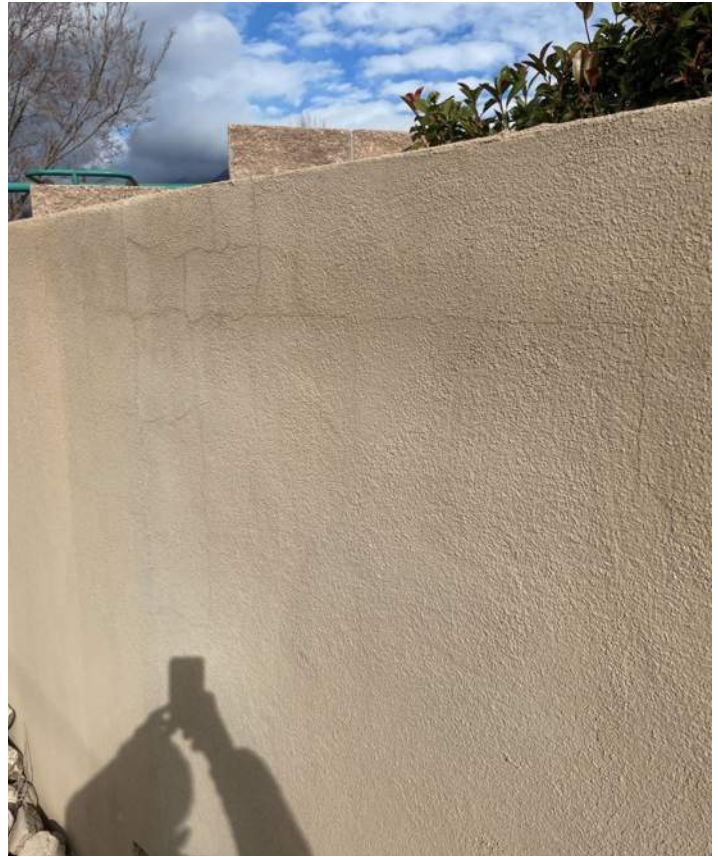
Hairline cracks can be repaired with a fog coat
